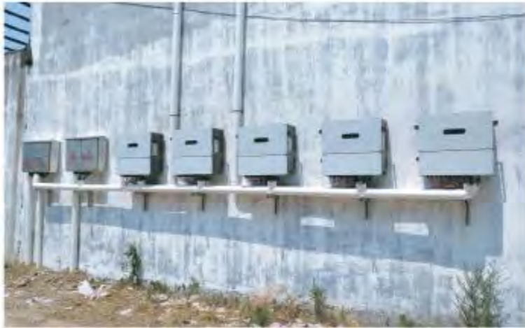
Rooftop PV Project in Shandong
