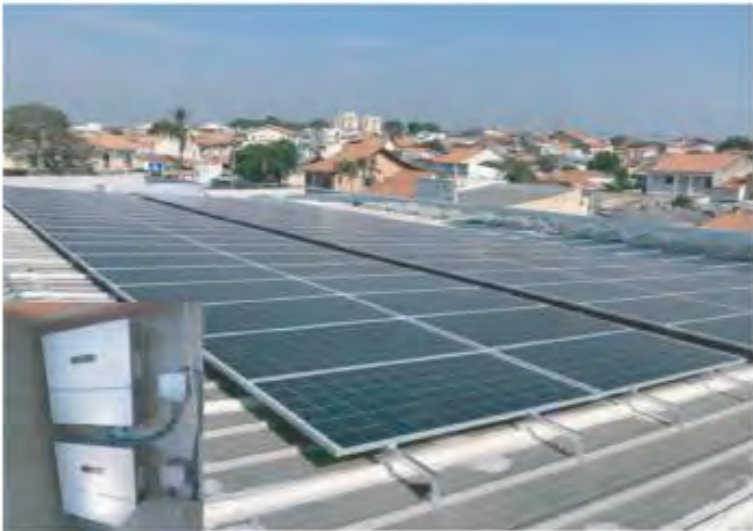
Brazil 500kW Rooftop Project
