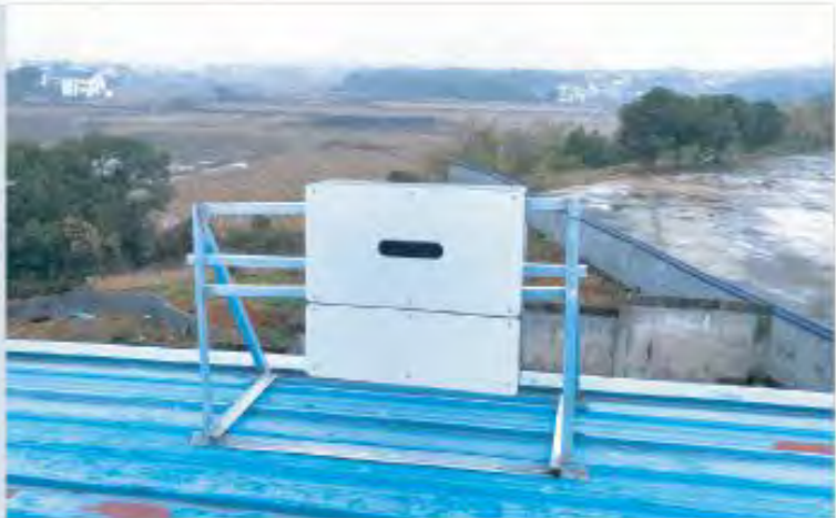
Roof-top PV Project in Hunan China
