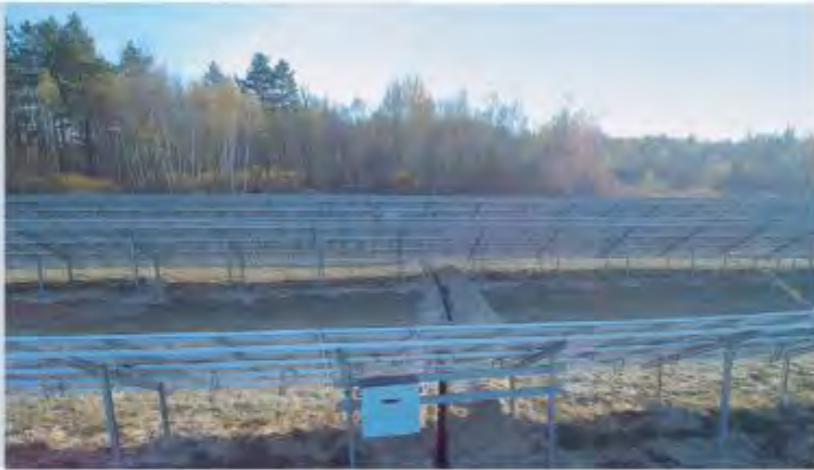
Ukraine 15MW Solar Plant
